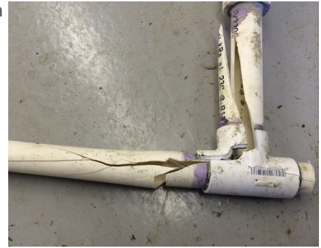
Figure 6-3: Broken PVC pipe from freeze damage.
