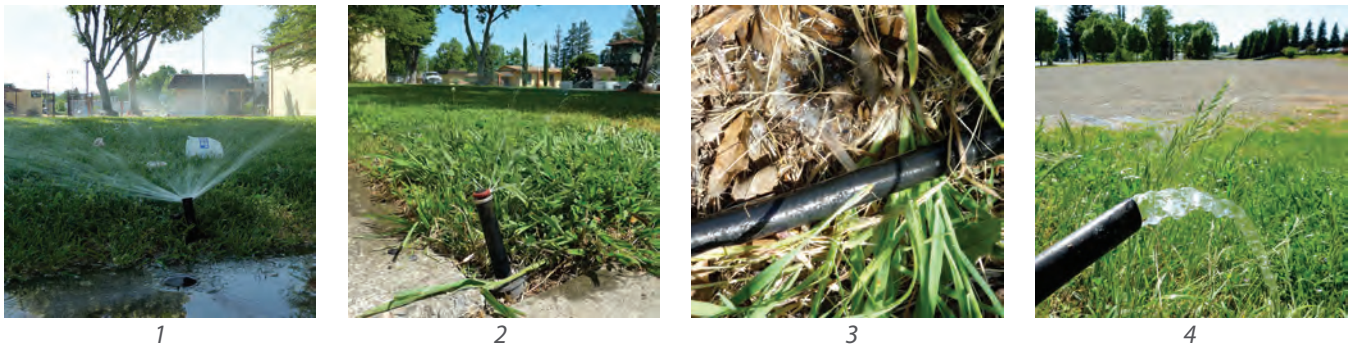
Figure 6-2: Left to right (1) (2) tilted sprinkler heads, (3) missing drip emitter, (4) severed drip line
