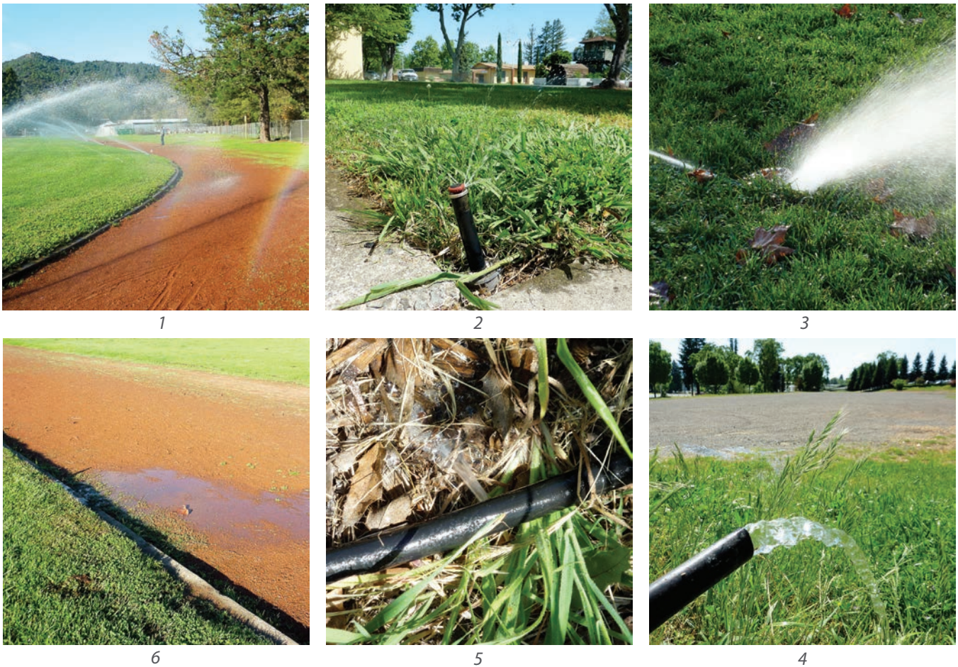
Figure 7-7: Clockwise (1) overspray, (2) tilted head, (3) head below grade, (4) severed drip line, (5) missing emitter, (6) leaking seals
