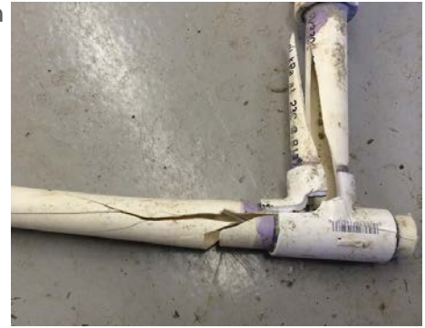
Figure 6-3: Broken PVC pipe from freeze damage.
