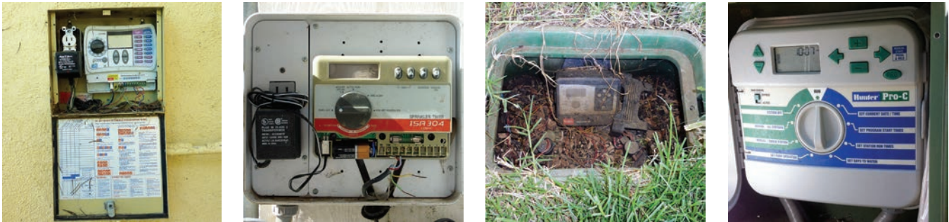
Figure 6-1: Various examples of controllers on location
