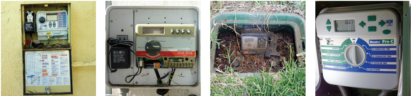
Figure 6-1: Various examples of controllers on location
